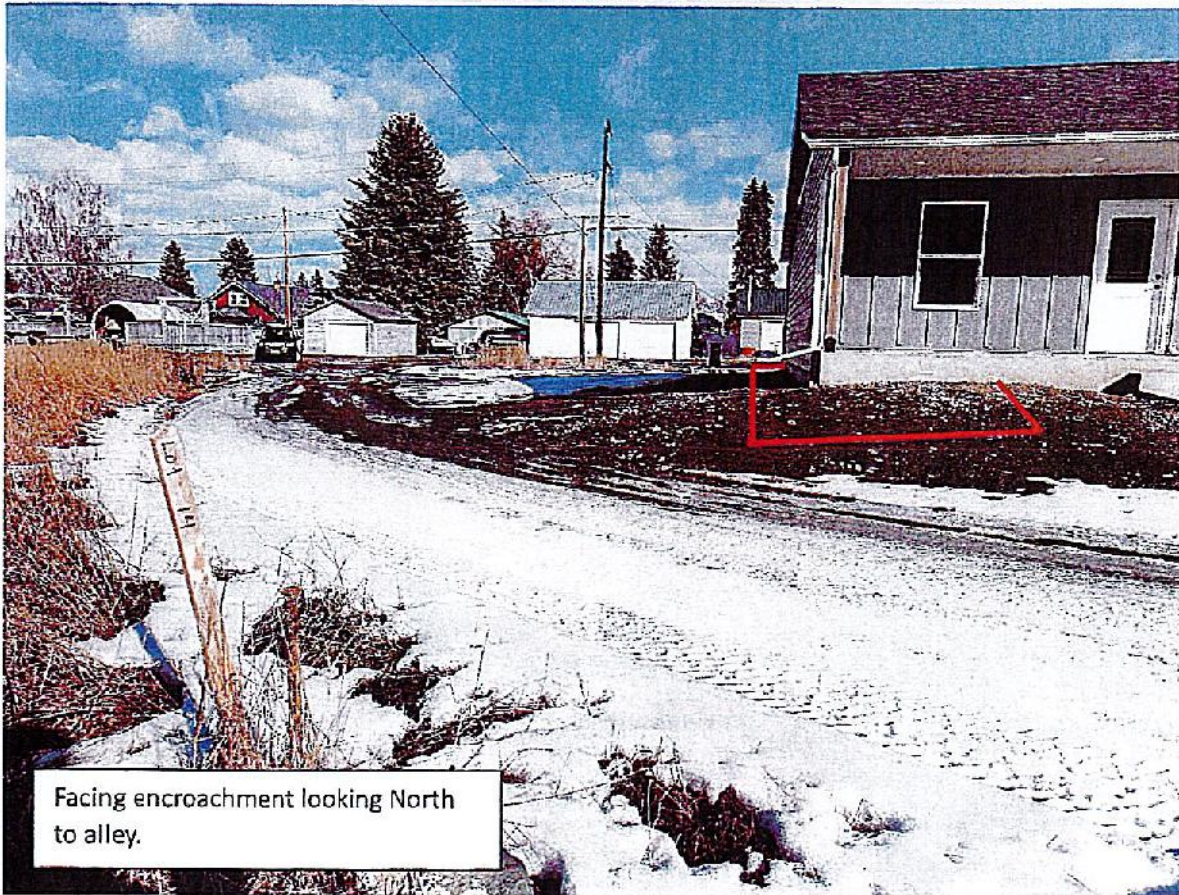
Facing encroachment looking North to alley.
